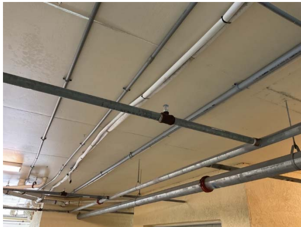
Fire suppression system head
