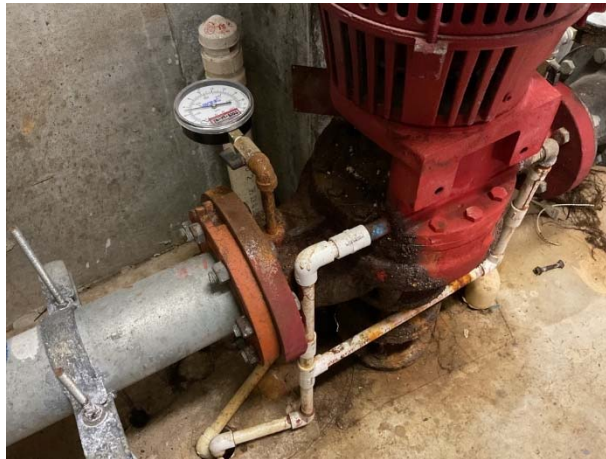
Fire suppression pump
