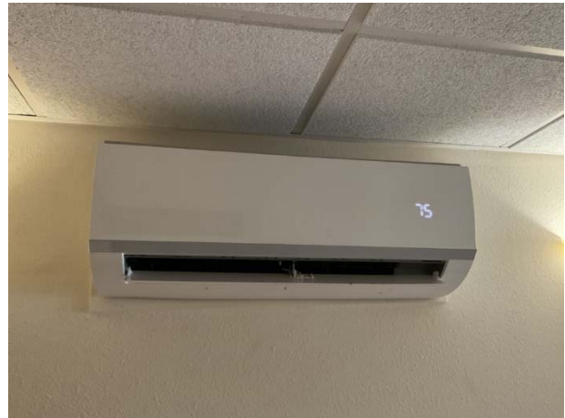
Mini-split system air handling unit
