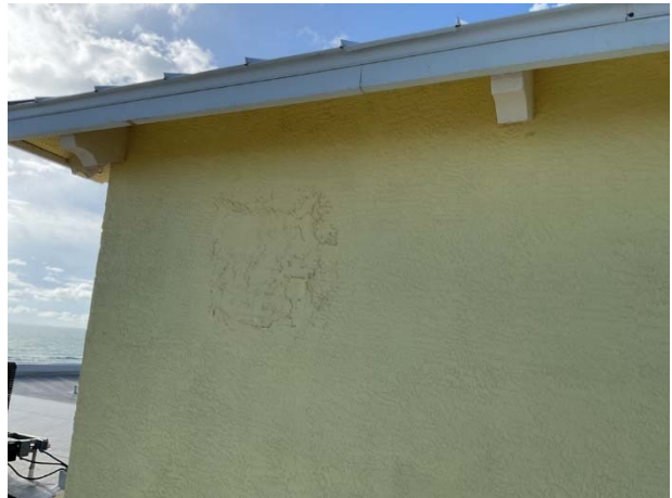
Stucco damage at the north elevator room
