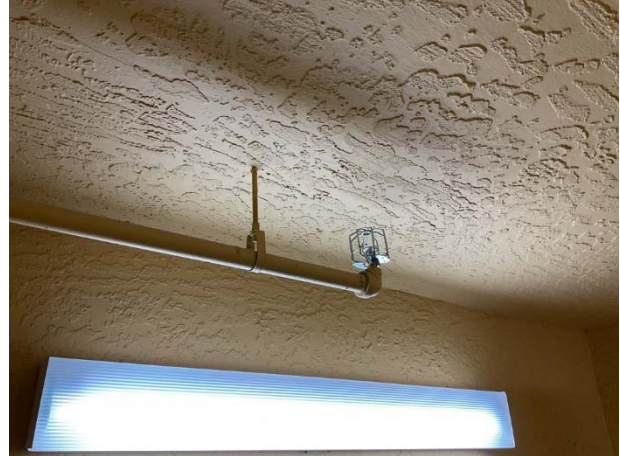
Fire suppression system sprinkler and emergency light fixture
