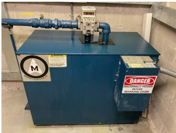
Hydraulic elevator equipment
