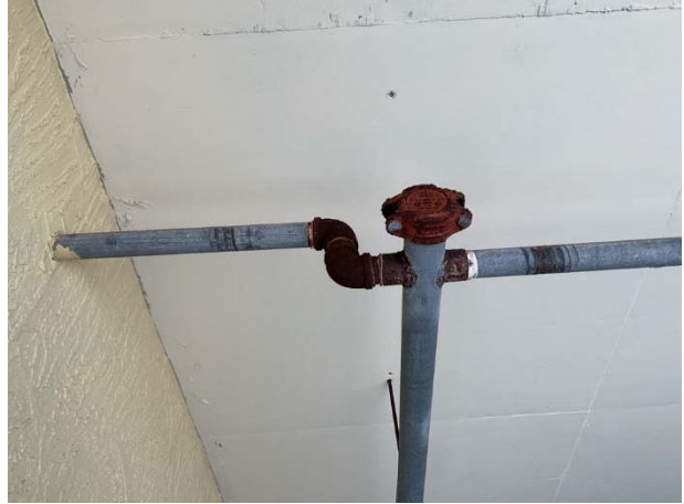
Rust at pipes
