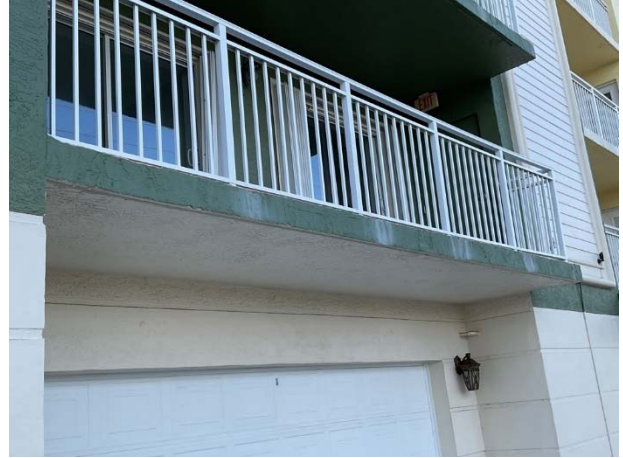
Edge spalls and efflorescence
