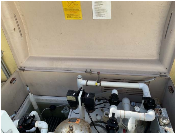
Pool mechanical equipment
