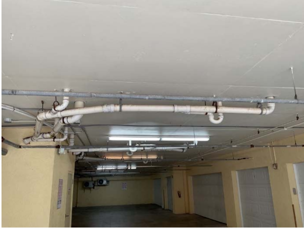
Fire suppression system
