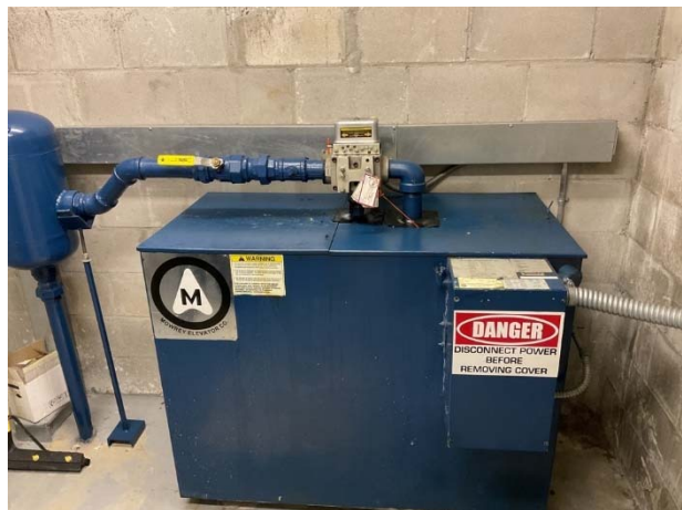
Hydraulic elevator equipment
