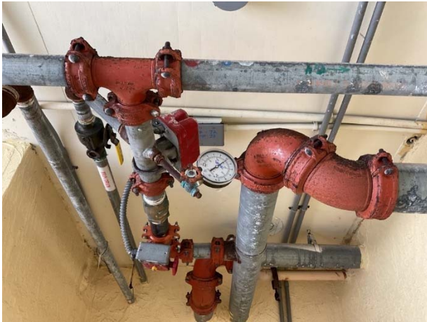
Rust at pipes
