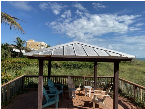
Metal roof deterioration
