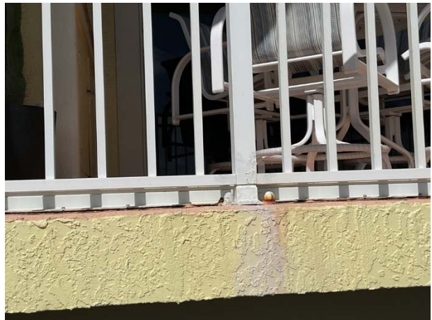
Rust at concrete connection
