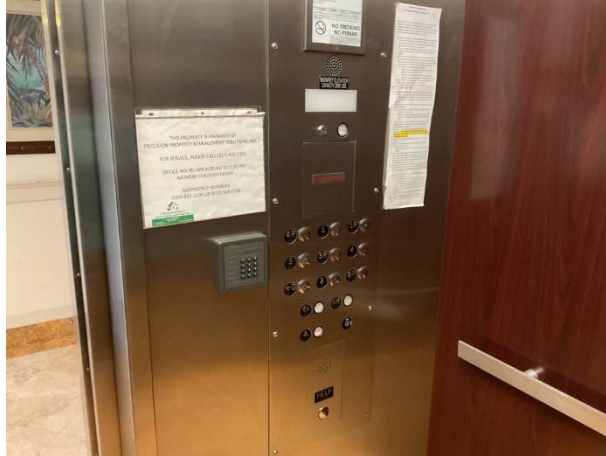
Hydraulic elevator controls
