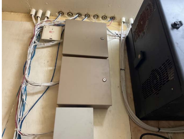
Access control system
