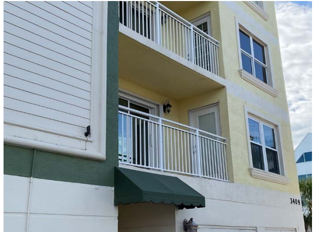
Bent railing section
