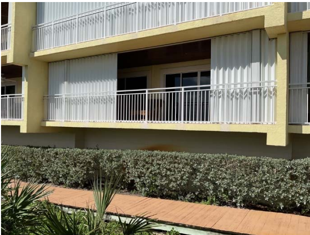
Efflorescence at railing attachment points
