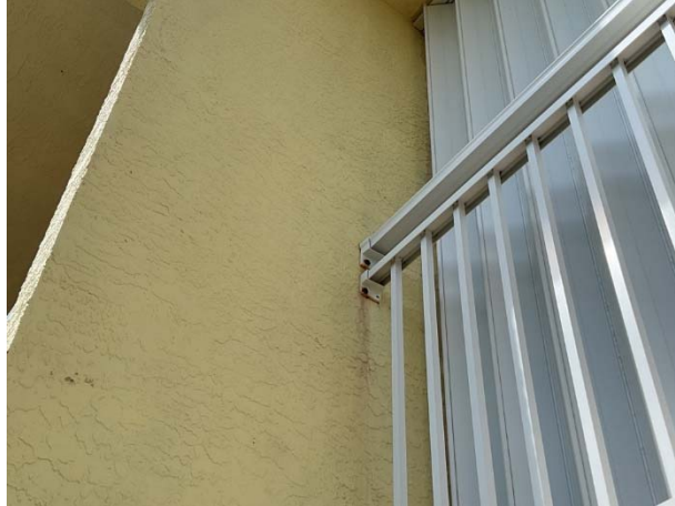
Rust at stucco connection
