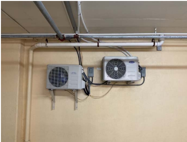
Mini-split system condensing units
